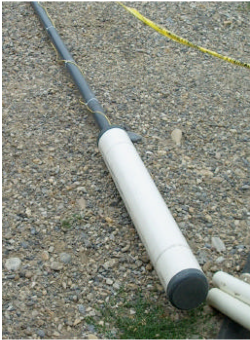
Photo 1 - Injection Well Screen and Riser
