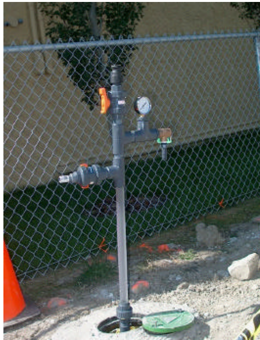
Photo 2 – A Wellhead Adaptor
