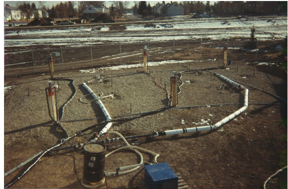
Figure 1. CFB Pilot Test Site
